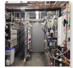
Purification inside the Containers
